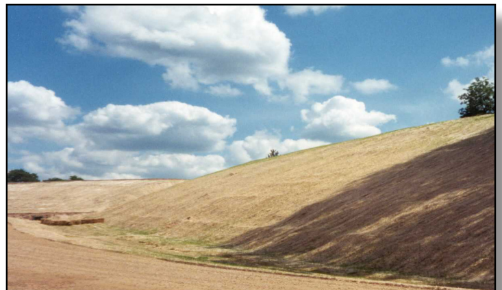
To assist in protecting slopes and allowing for vegetation reclamation, temporary ECBs can be used to stabilize slopes and channels.
